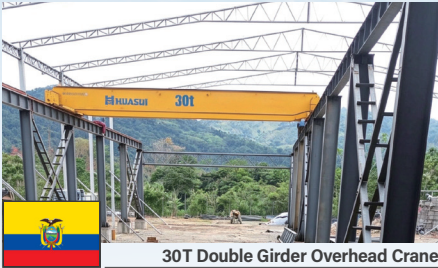
30T Double Girder Overhead Crane
