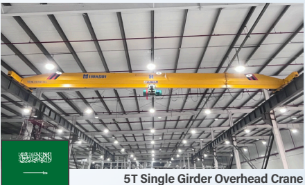
5T Single Girder Overhead Crane
